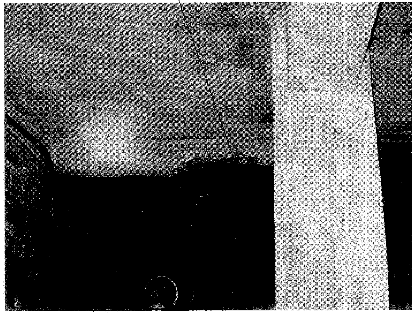
PHOTO 3: SPALL AT THE UNDERSIDE OF EXISTING CONCRETE BEAM IN BASEMENT
