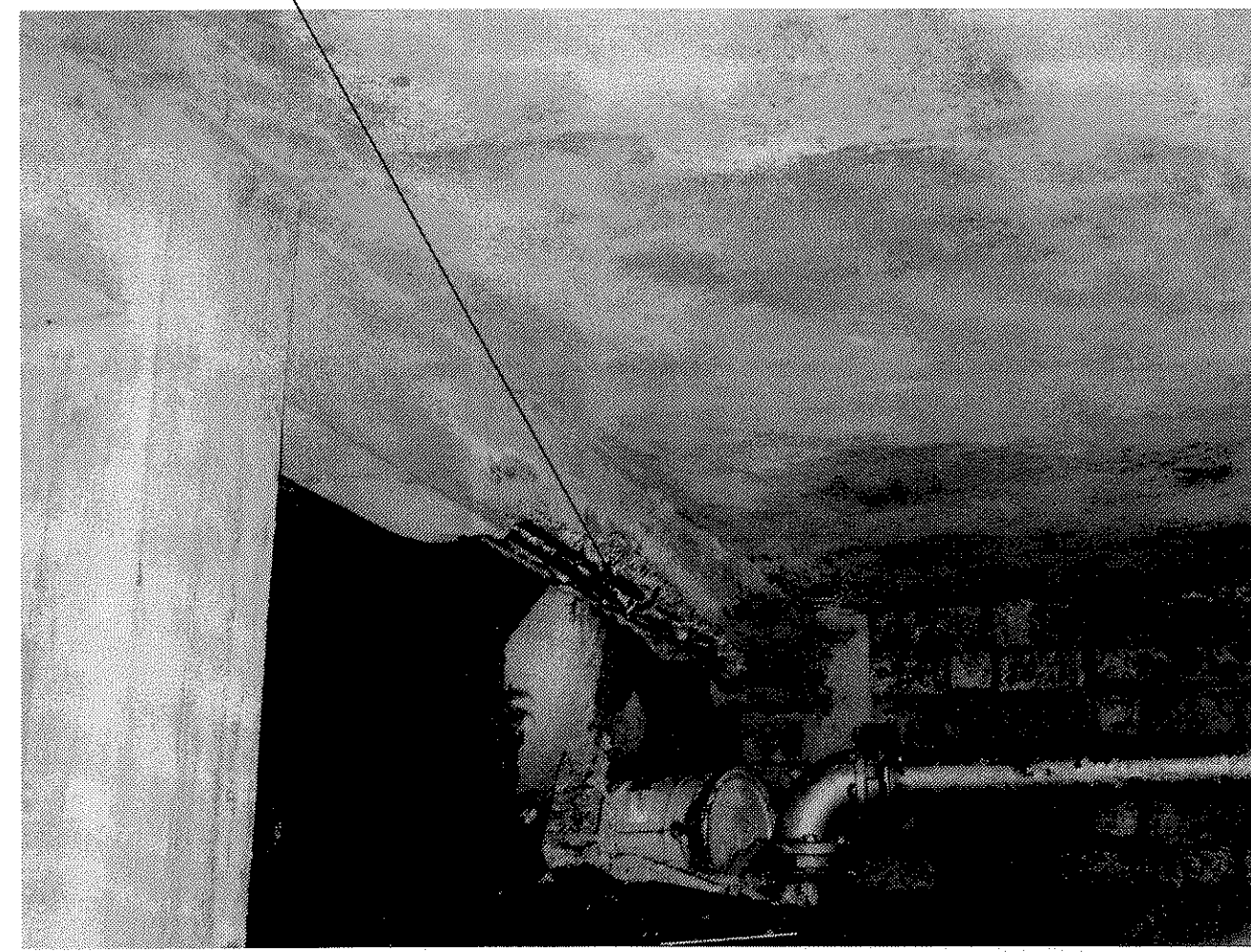
PHOTO 2: SPALL AT THE UNDERSIDE OF EXISTING CONCRETE BEAM IN BASEMENT
