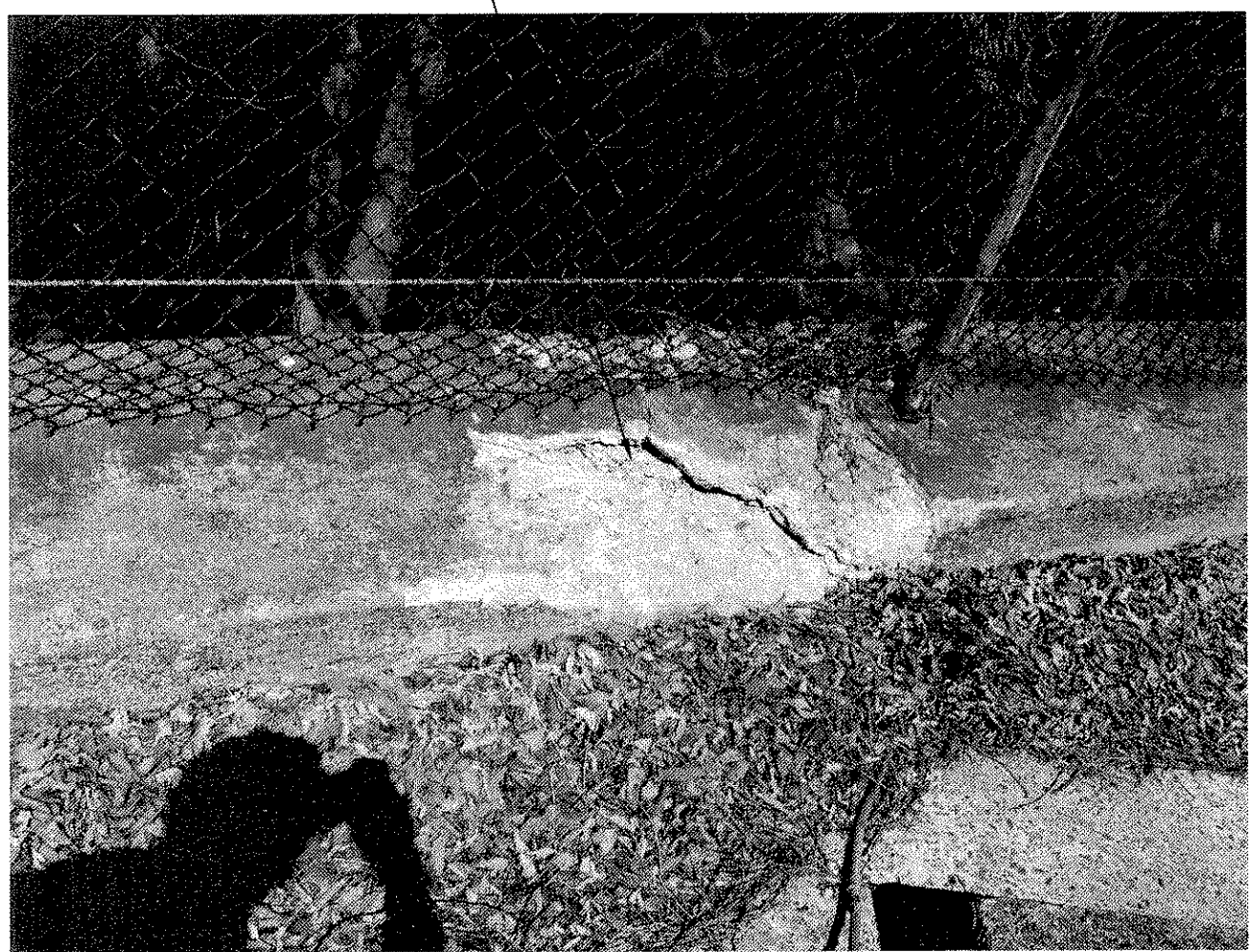
PHOTO 1: SPALL AT TOP OF EXISTING RETAINING WALL
